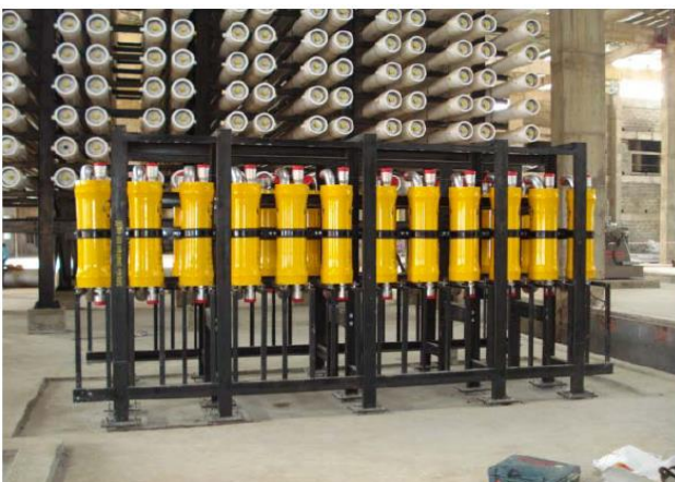
RO Process Unit, Pressure vessels & Energy Recovery System
