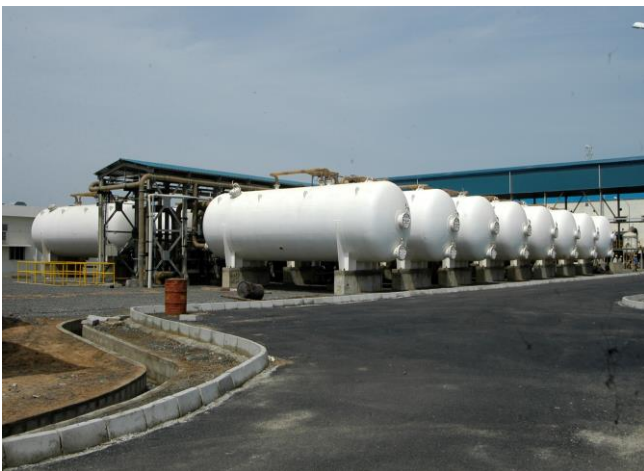
Pre-treatment Pressure Filter Vessels
