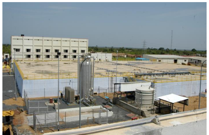
Post-Treatment CO2 Dosing unit
