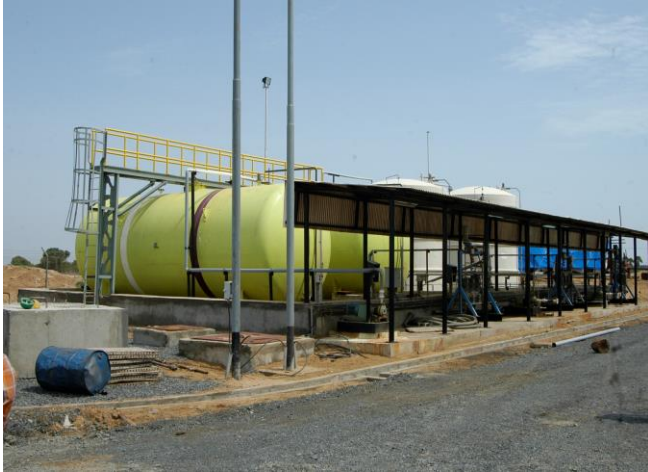
Chemical Dosing unit for Pre-Treatment
