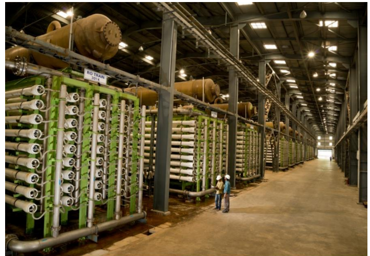
Reverse Osmosis (RO) Section.
